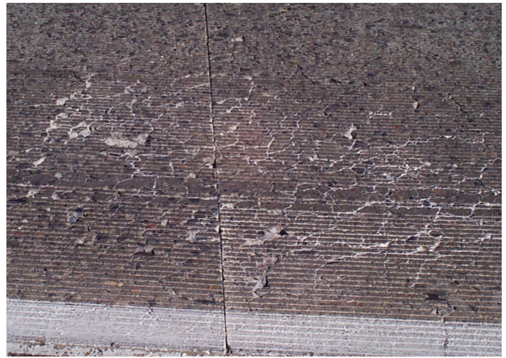
Figure 1. An example of ASR-related map-cracking in concrete pavement (Photo Credit L. Sutter)
