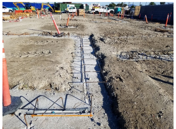
Figure 15. Completed foundation on cement-treated subgrade (©2020 Pavement Recycling Systems, Inc., used with permission)
