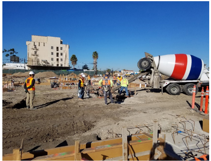
Figure 14. Constructing foundation for the school structure (©2020 Pavement Recycling Systems, Inc., used with permission)
