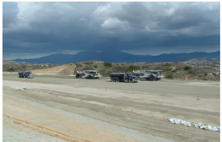
Figure 11. Reclaimers mixing the subgrade and cement (Jeff Wykoff, California Nevada Cement Association, used with permission)
