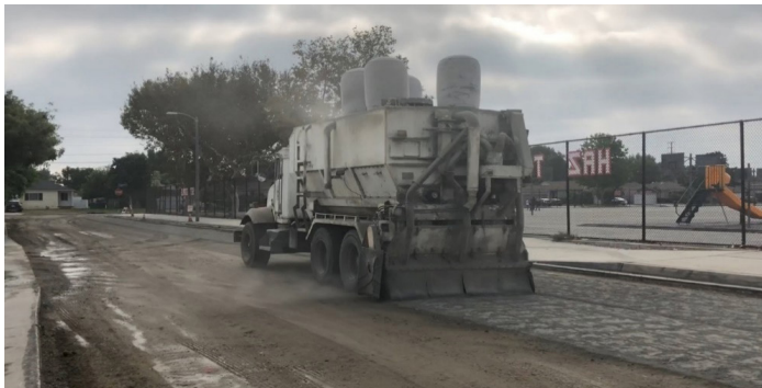
Figure 5. Spreader truck during portland cement application (©2020 Pavement Recycling Systems, Inc., used with permission)
