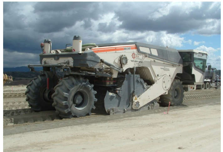
Figure 7. Mixing portland cement and native soil with a reclaimer (Jeff Wykoff, California Nevada Cement Association, used with permission)
