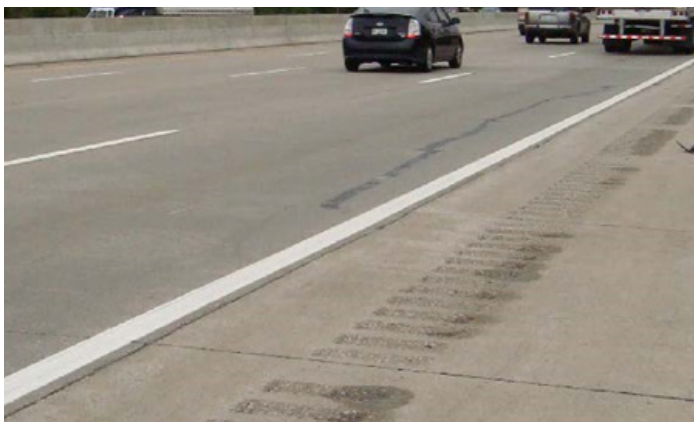
Figure 2. Longitudinal cracking attributed to erosion of interlayer
