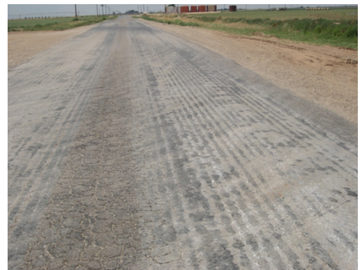
Figure 2. Rural road with extreme fatigue cracking due to shale gas exploration
