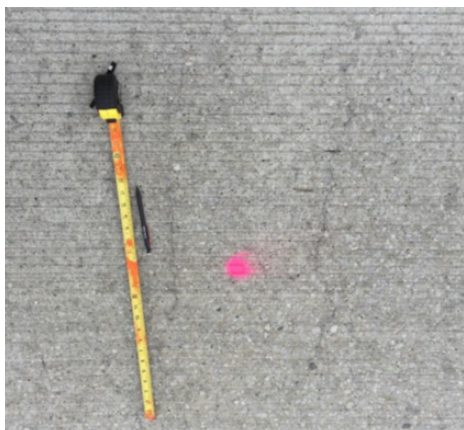
Figure 9. Cracking on southbound inner lane of the normal concrete deck
