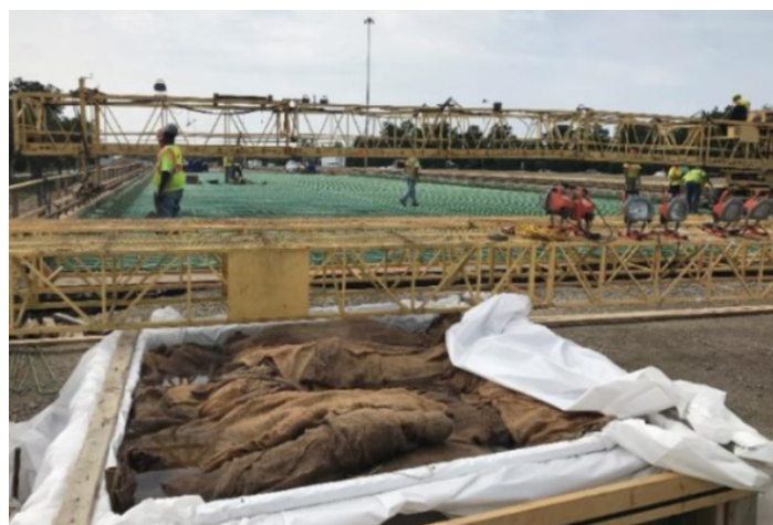
Figure 2. Bridge prior to deck placement, with wet burlap ready to be placed
