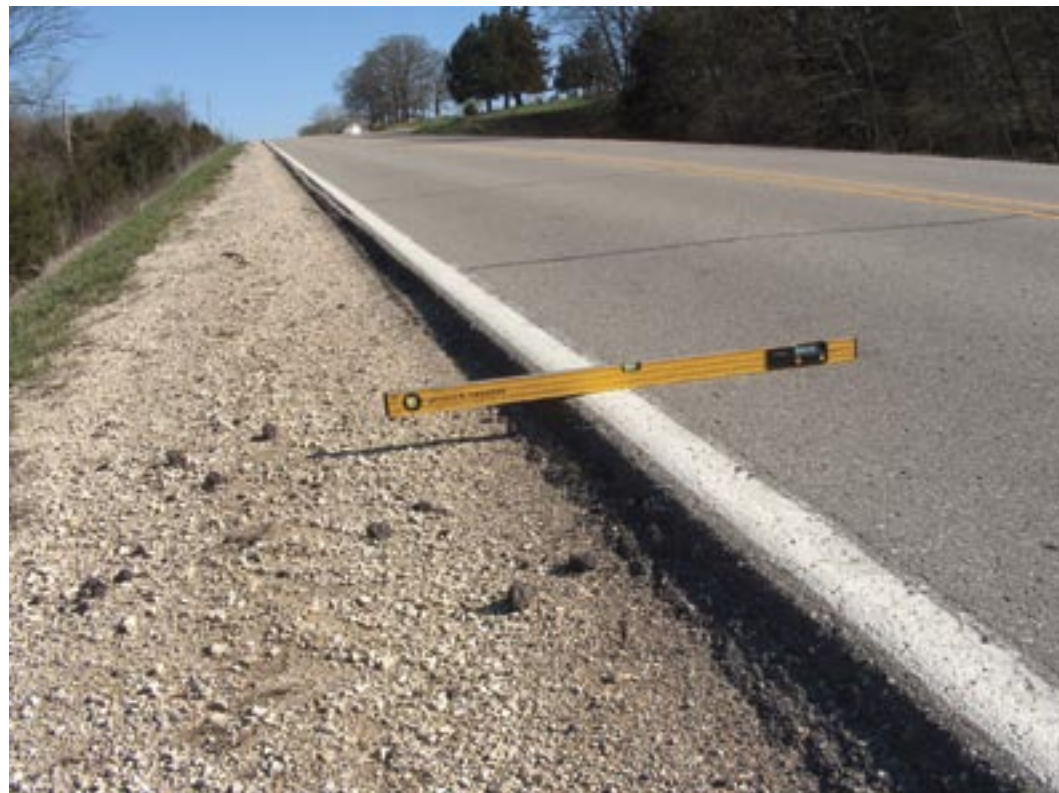
Figure 5-1. Drop-off on a significant grade due to erosion
