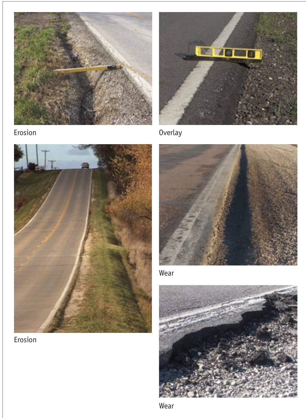
Figure 1-1. Common causes of pavement edge drop-off
