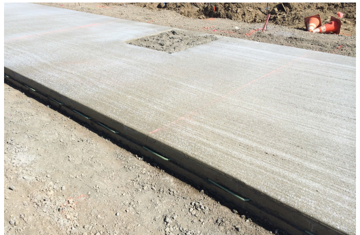
Figure 5. Inadequate curing compound application
