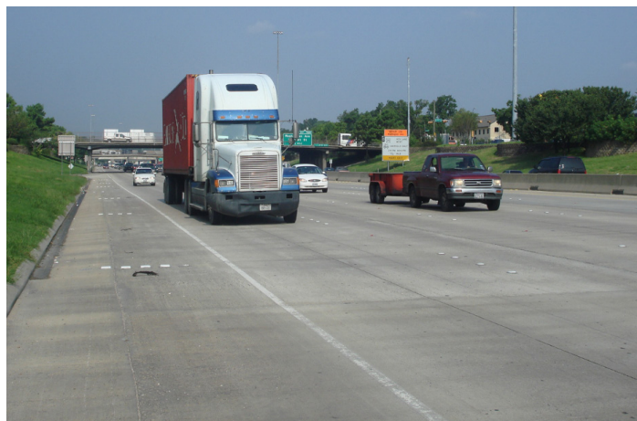
Figure 4. I-10 near Houston, TX in 2006 after 11 years of service (photo source: Prof. Moon Won)
