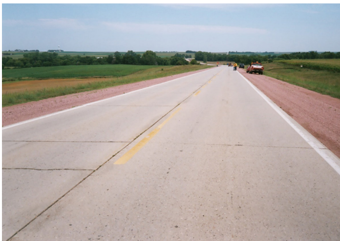
Figure 3. U.S. 75 near Rock Rapids, IA in 2006 after 40 years of service and some rehabilitation
