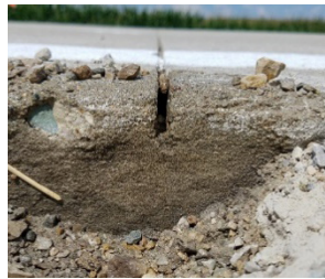
Figure 22: Lack of crack deployment at a sawed contraction joint
