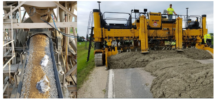
Figure 3. Mitchell County test section construction showing addition of fibers at the batch plant and overlay paving
