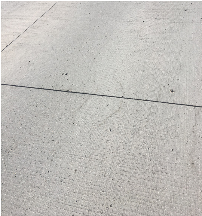
Figure 7. North Dakota SPS-2 field visit, cracking over dowels
