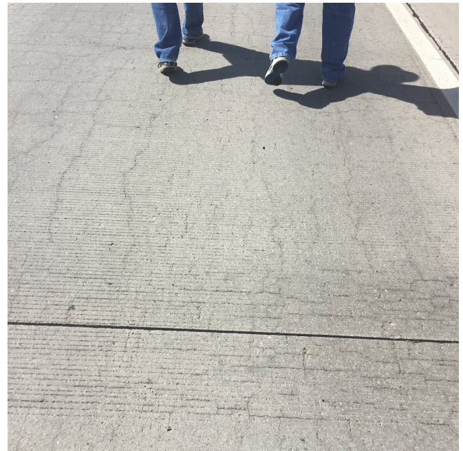
Figure 5. Kansas SPS-2 field visit, 900 psi surface cracking
