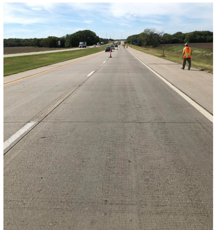
Figure 6. Kansas Section 0209 (8 in. PCCP on 4 in. PATB and 4 in. DGAB, 550 psi mix, 12 ft. shoulder)
