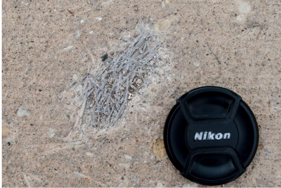
Figure 3.3. Example of fiber balling in a hardened BCOA application in a parking lot, shown with a lens cap 60 mm in diameter
