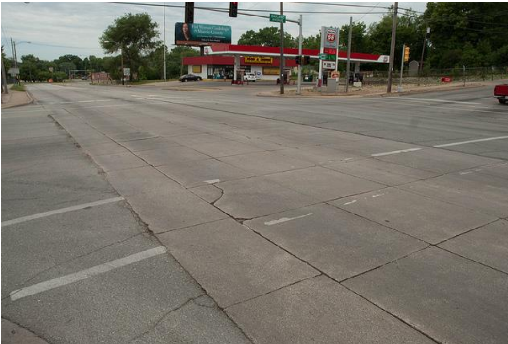
Figure 5.5. Example of slab migration in BCOA without macrofibers
