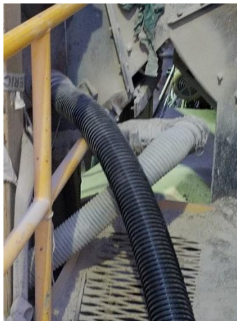
Figure 6-3. Connection of fiber and ECR-GTR hoses at similar location near bottom of drier drum
