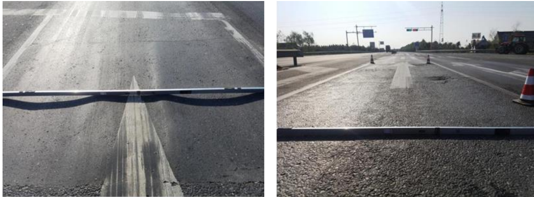
(a) Rutting in asphalt concrete
