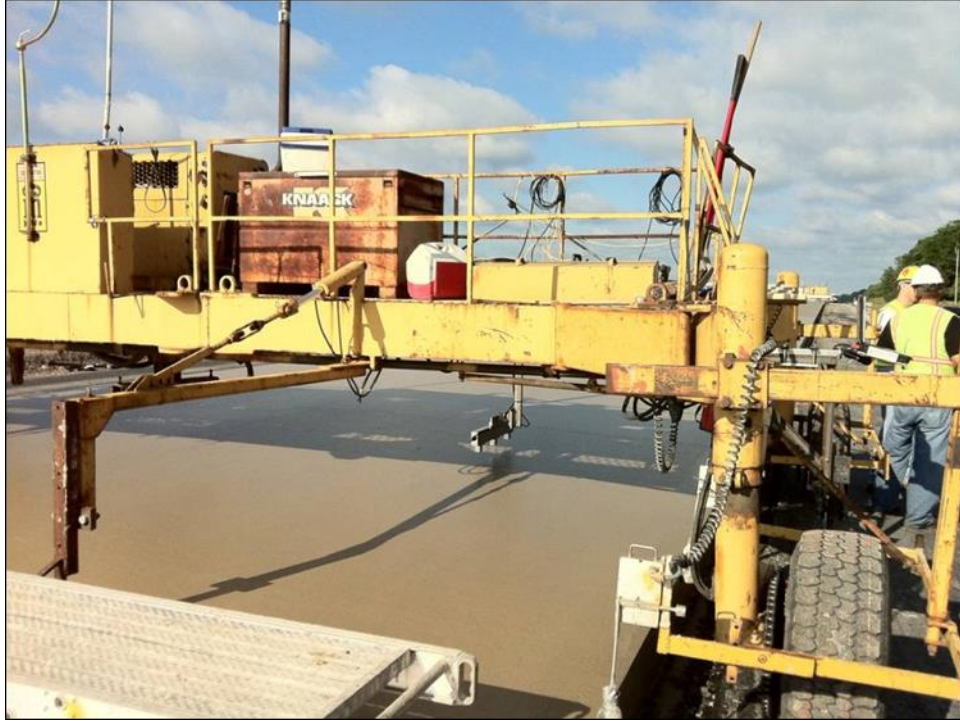
Figure 20. RTP equipment mounted to a work bridge during the SHRP2 New York demonstration
