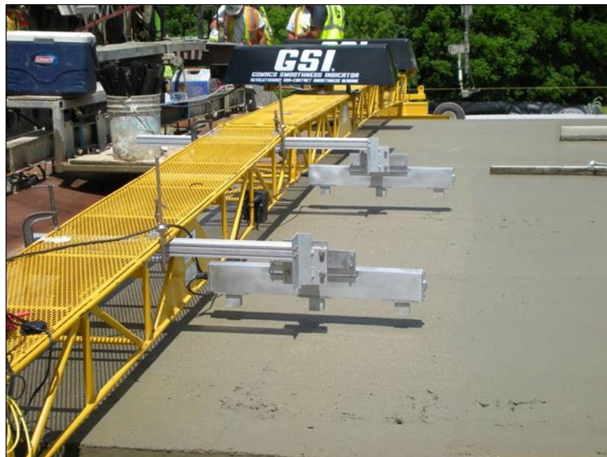
Figure 22. GOMACO GSI and Ames RTP mounted to a work bridge towed by the paver
