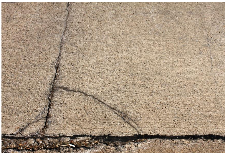
Figure 11. A corner crack likely due to loss of support due to curling
