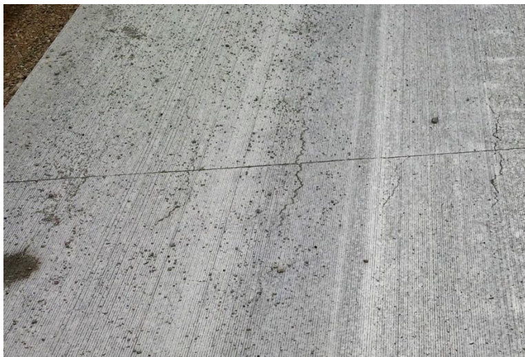
Figure 10. Cracks in a pavement, likely a combination of plastic shrinkage and settlement effects over dowels
