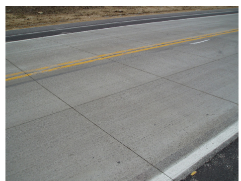
c) Route D current pavement condition (2017)
