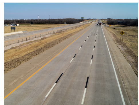
c) I-40 Current pavement condition (2017)
