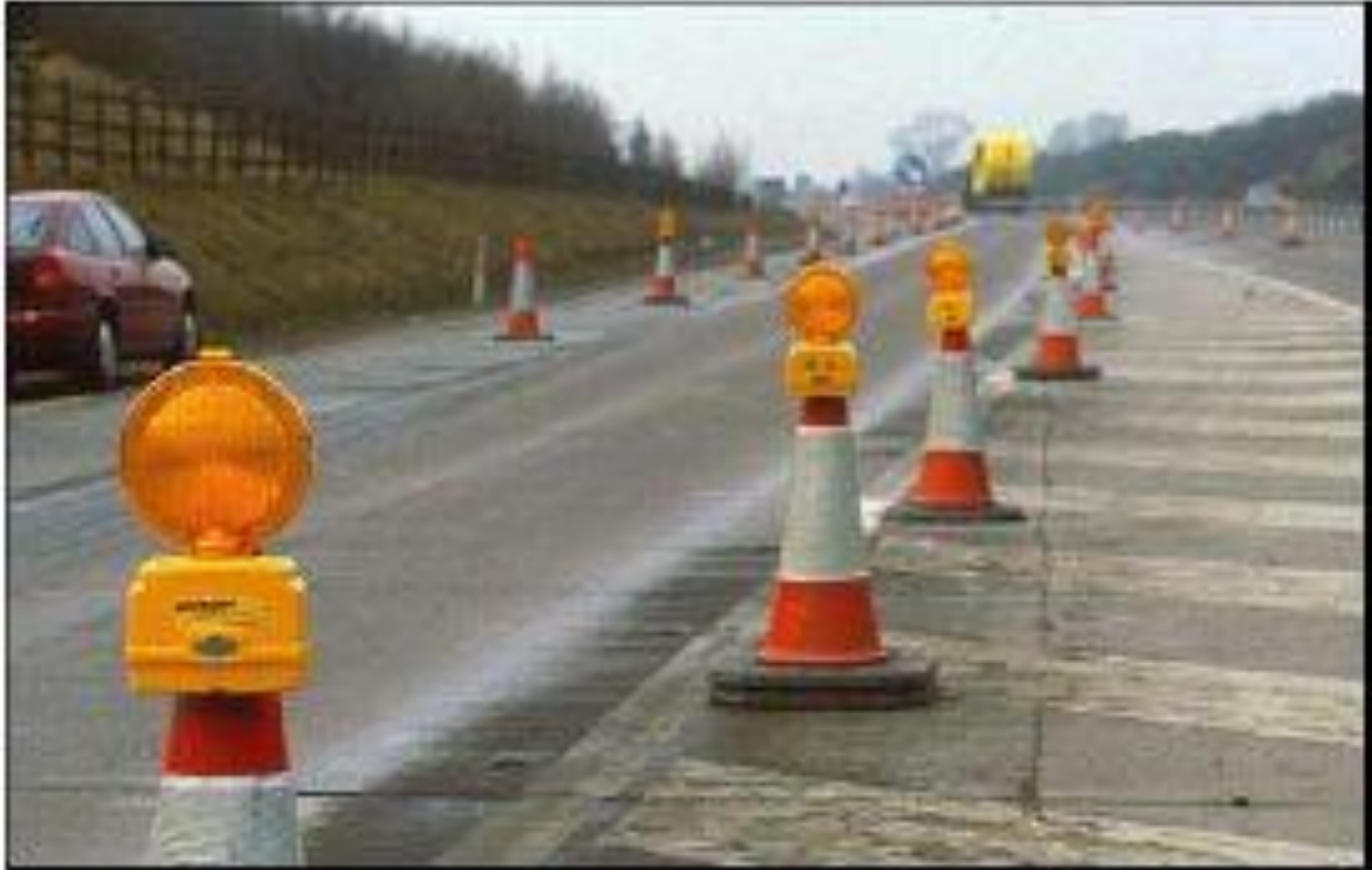
FIGURE 2 Sequential warning light (HA, 2005b).
