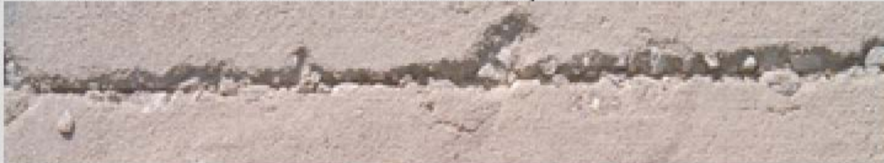
C. UNACCEPTABLE RAVELING – Sawn too early
