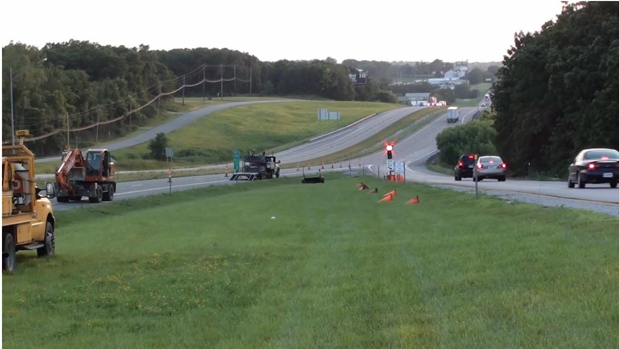
Figure 2.6 I-70 WB at mile marker 131, three-head signal.
