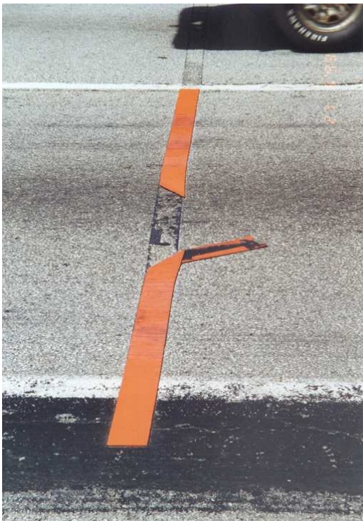
FIGURE 4-19 Worst material loss after eight days.
