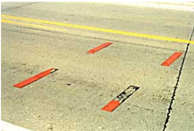
FIGURE 2-33 Damaged rumble strips – Site B.
