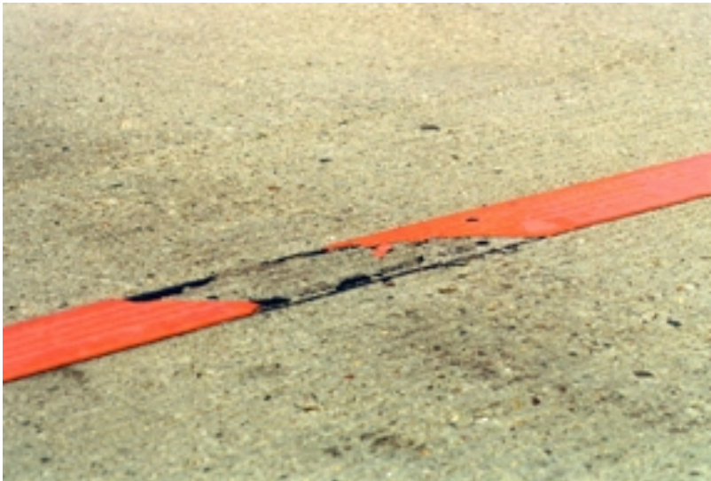
FIGURE 2-34 A damaged rumble strip – Site B.
