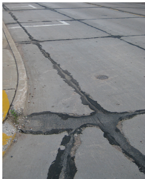
Figure 1: Typical distress in a city street
