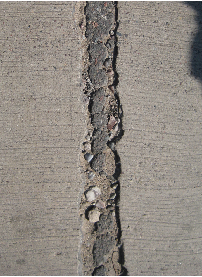
Figure 3: Cracks formed at inch increments from sawn face
