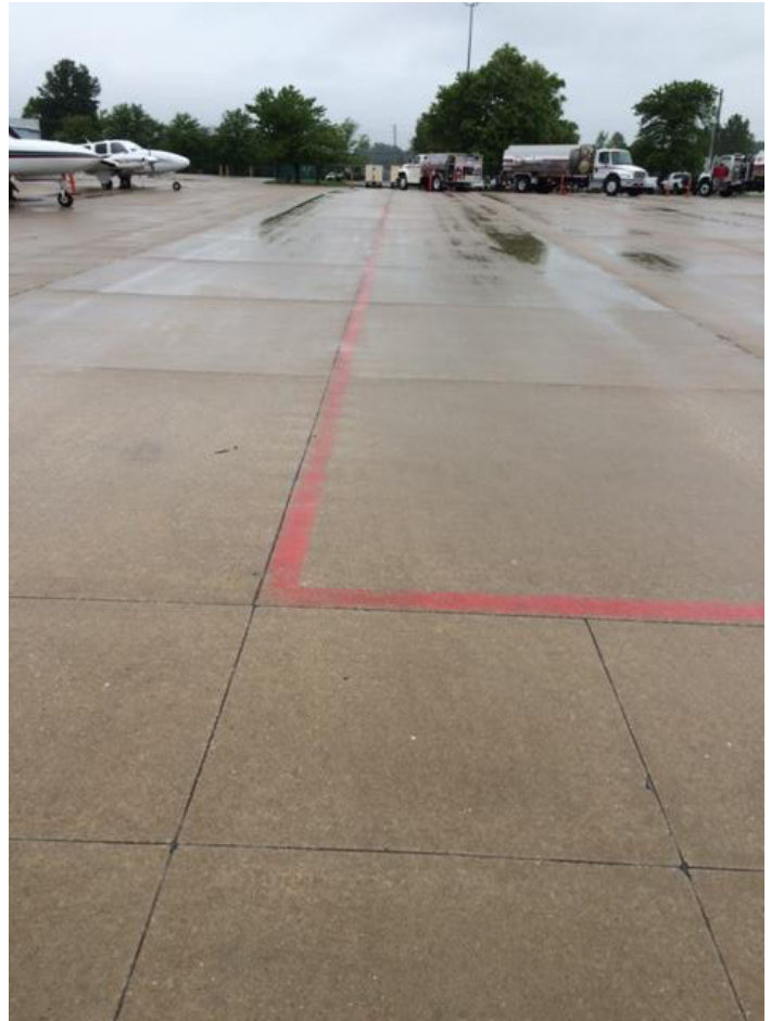
Figure 5. Current pavement condition (June 2015)
