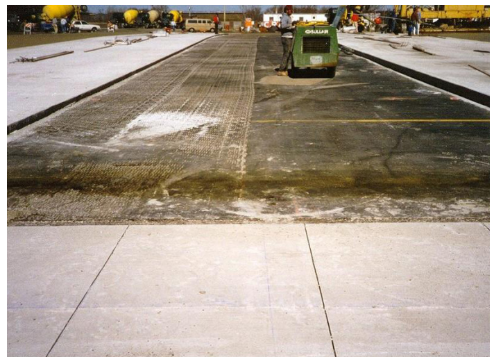
Figure 2. Photo from original construction of the concrete overlay at Spirit of St. Louis Airport in 1994
