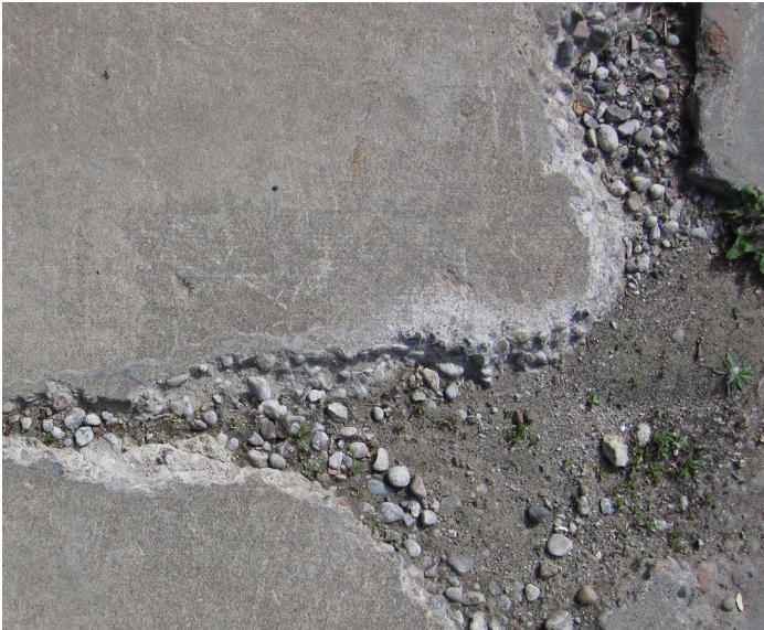
Figure 3. Example of paste disintegration
