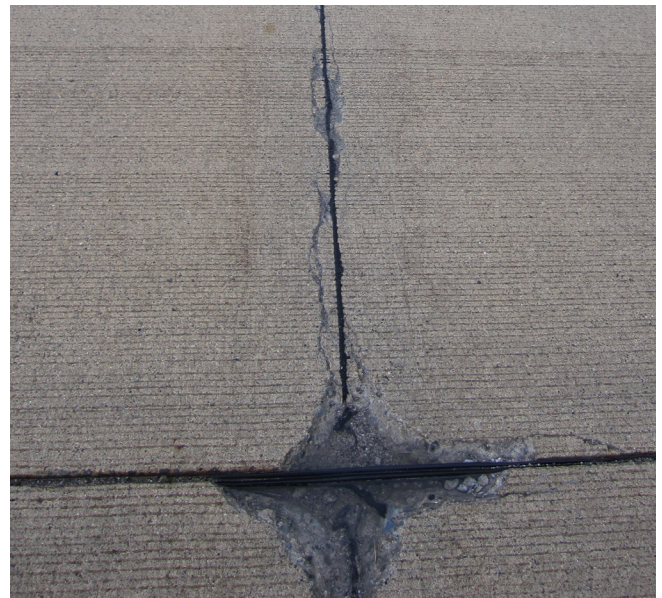
Figure 1b. Progression of joint deterioration
