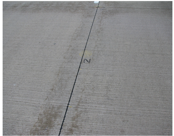
Figure 1a. Initial stage of joint deterioration
