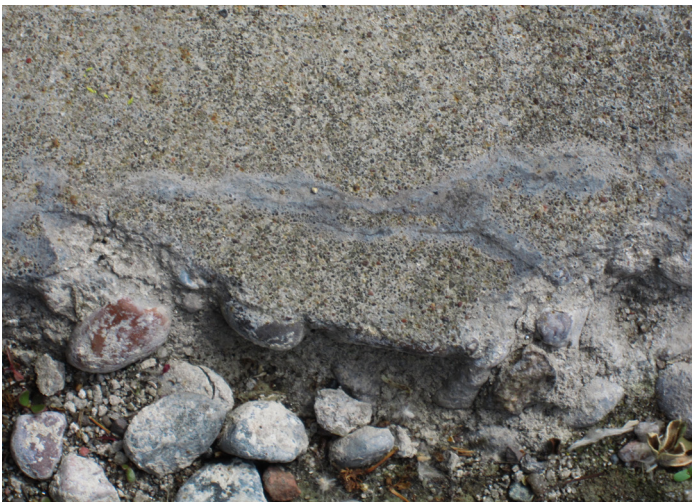
Figure 4. Exudate visible along cracks parallel to the deterioration front
