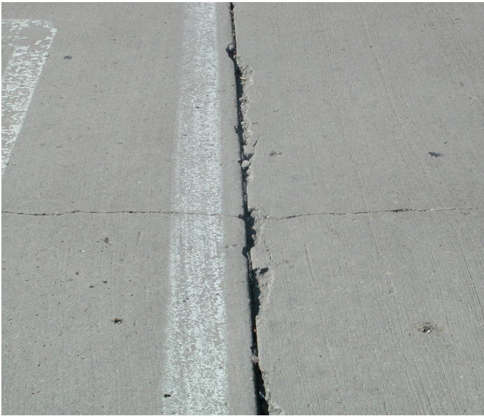
Figure 2b. Further progression of joint deterioration showing loss of larger wedges
