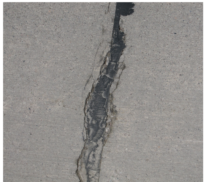
Figure 2a. Further progression of joint deterioration showing loss of thin flakes
