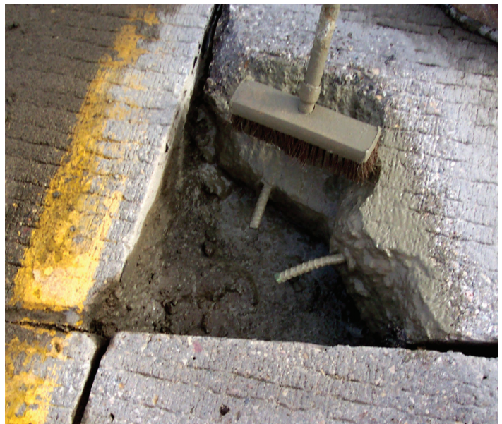
Figure 4. Deteriorated pavement corner where Type 3 repair can be used. As shown in photo, tie rods are drilled at an angle into existing slab and then bent straight to tie the new patch with the existing pavement (strips of compressible material are positioned prior to placement of patch material).
