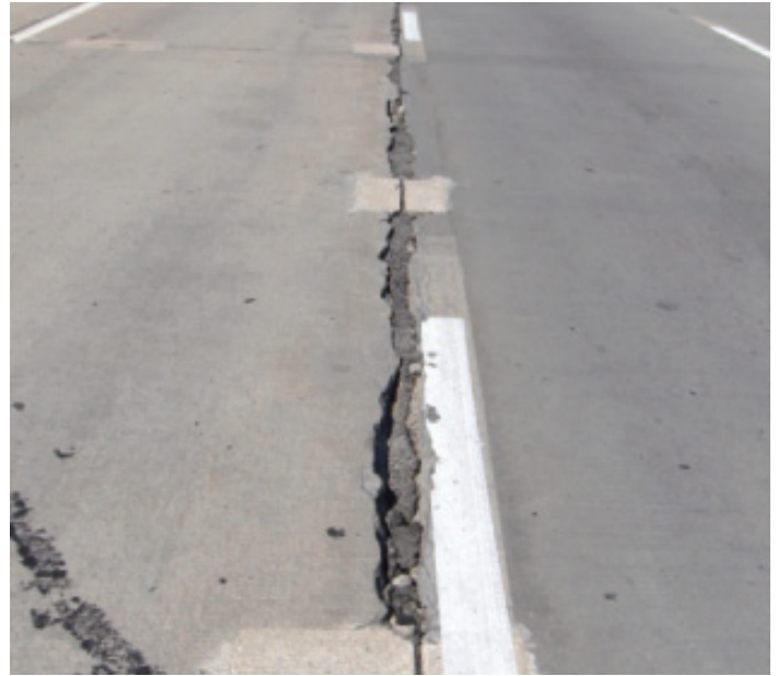
Figure 3. Longitudinal joint deterioration where Type 2 repair can be used
