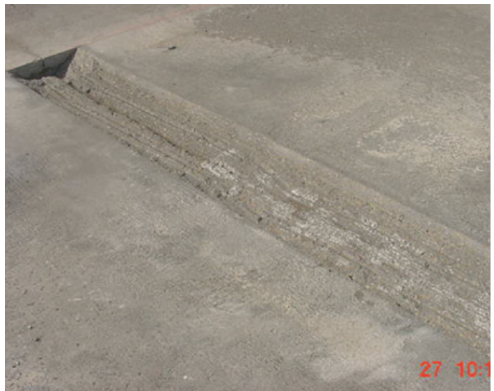
Figure 6. Type 2 repair—milling (a strip of compressible material is positioned prior to placement of patch material)
