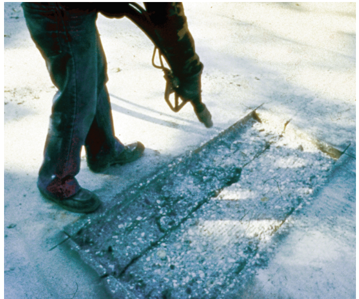
Figure 5. Type 1 repair—sawing and chipping (a strip of compressible material is positioned prior to placement of patch material)
