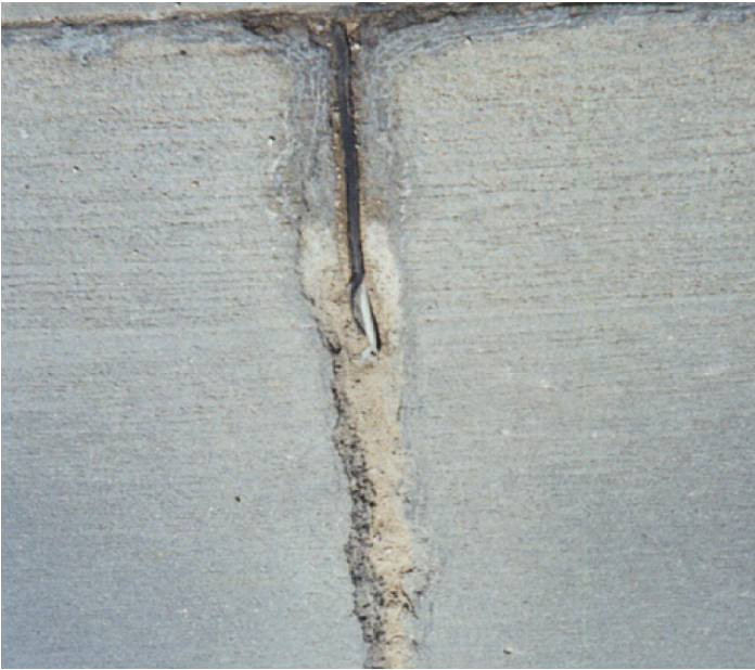
Figure 2. Spot repair required
