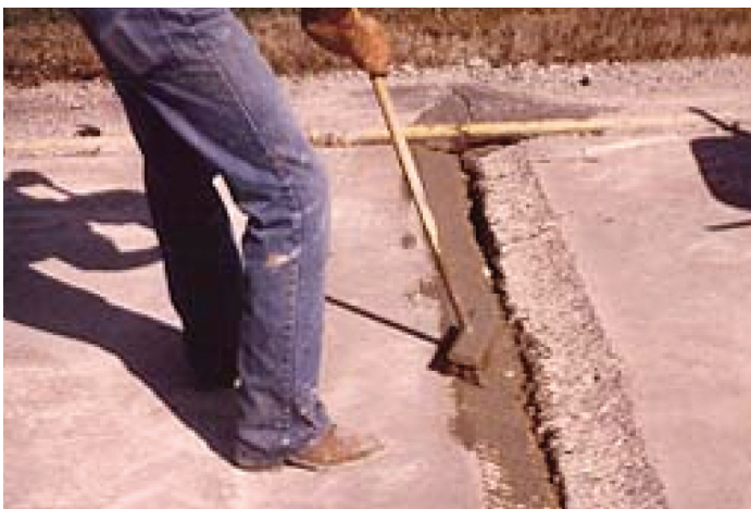
Figure 8. Placement of cement grout as bonding agent (a strip of compressible material is positioned prior to placement of patch material)
