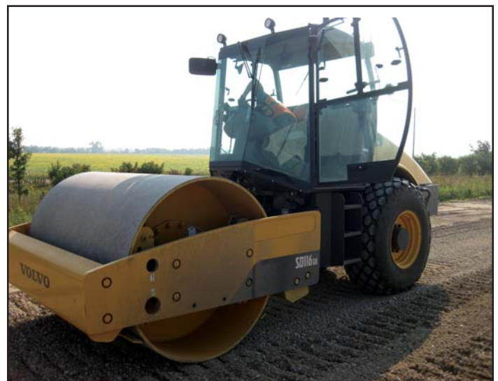
Figure 2. Volvo SD116DX roller with onboard Trimble CB430 display unit used on I29 project in Monona County, Iowa
