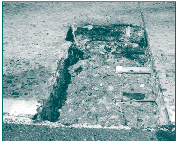
Figure 11. Corroded (and non-corroded) dowels at in-service pavement joint (photo credit: Washington State DOT Pavement Guide)
