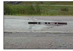
Figure 1. Deteriorated pavement that is a good candidate for FDR
