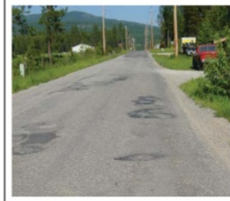
Figure 1. Deteriorated asphalt pavements that are candidates for full-depth reclamation with cement
