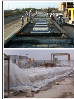
Figure 1. Precast concrete pavement panels are produced and cured in a controlled environment (steam curing [bottom] is not required but is an option for some precasters).
