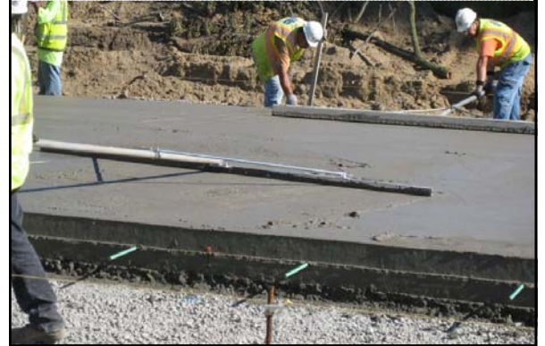
Stringline Sensor Moved off Line
