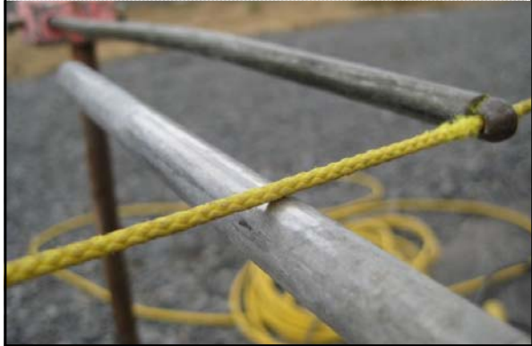
Stringline Sensor Moved off Line
