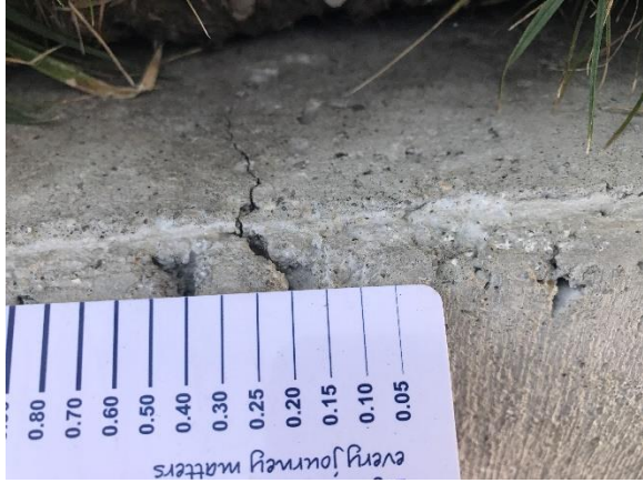
Figure 66. Joint 9 in the IC section
