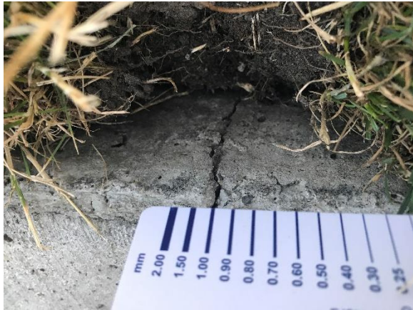
Figure 67. Joint 10 in the IC section
