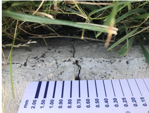
Figure 61. Joint 4 in the IC section
