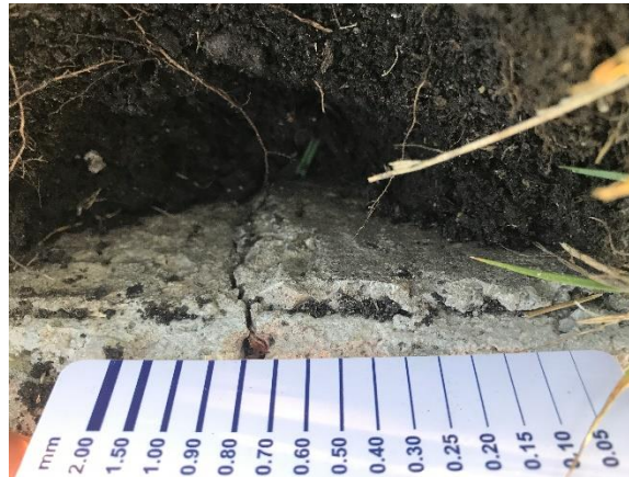
Figure 58. Joint 1 in the IC section
