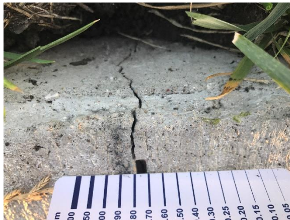
Figure 62. Joint 5 in the IC section
