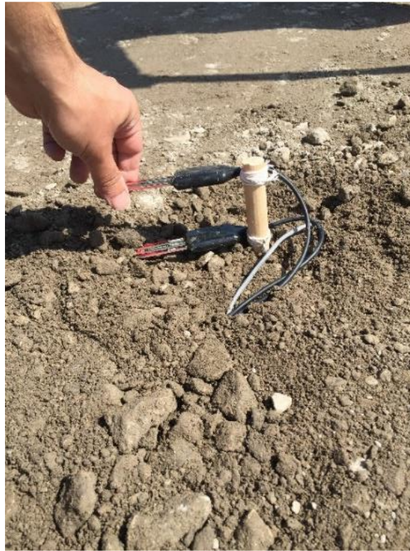
Figure 12. Installation of Decagon 5TE sensors at the top and bottom layers of JPCP
