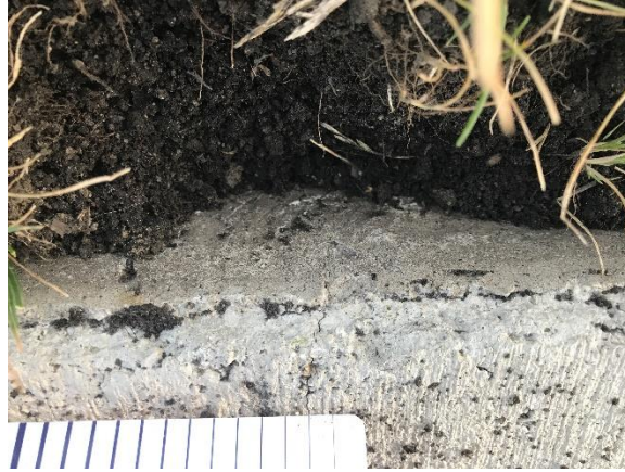
Figure 60. Joint 3 in the IC section
