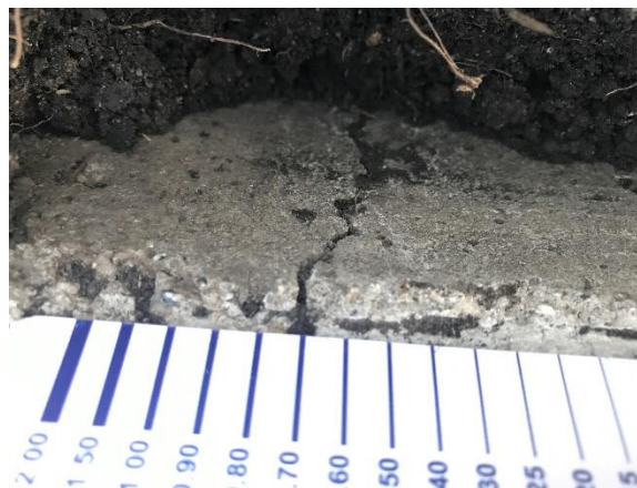
Figure 59. Joint 2 in the IC section
