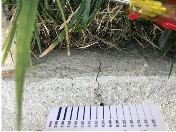
Figure 64. Joint 7 in the IC section
