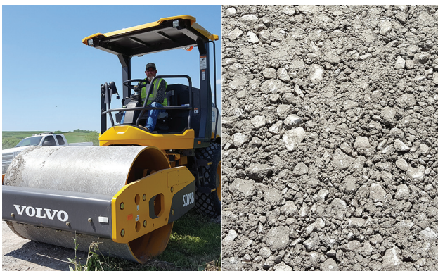
Compacting the new granular-surfaced road layer with a vibratory smooth drum roller (left), and bentonite-treated surface material after compaction (right)
