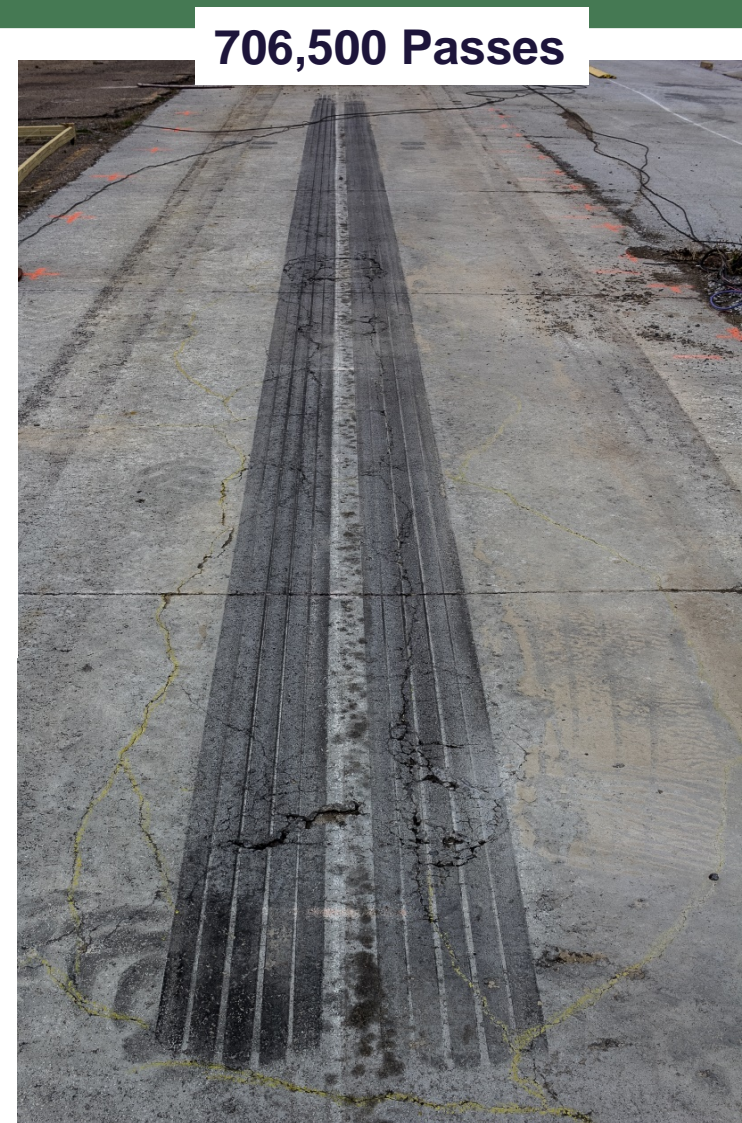
Pavement Condition at the end of testing
