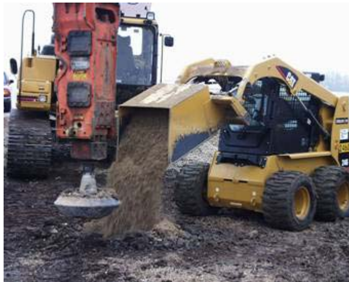
Figure 5.5. High-energy, low-frequency hammer used for the construction of Geopier foundations [photo courtesy of the Iowa DOT].
