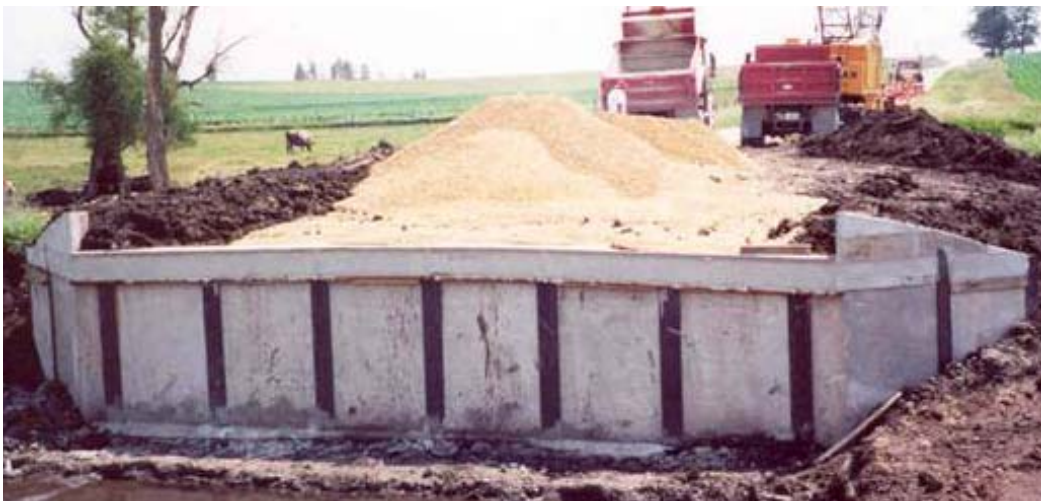
Figure 3.4. Stub abutment system with a precast concrete panel backwall [photo courtesy of Black Hawk County, Iowa].
