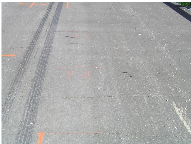
Figure 5.3. Transverse cracking, Span 1, one year post construction
