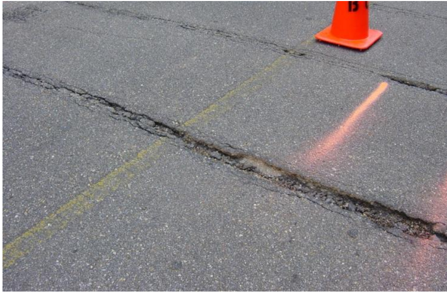
Figure 2.1. Wearing surface deterioration resulting from cupped deck panels
