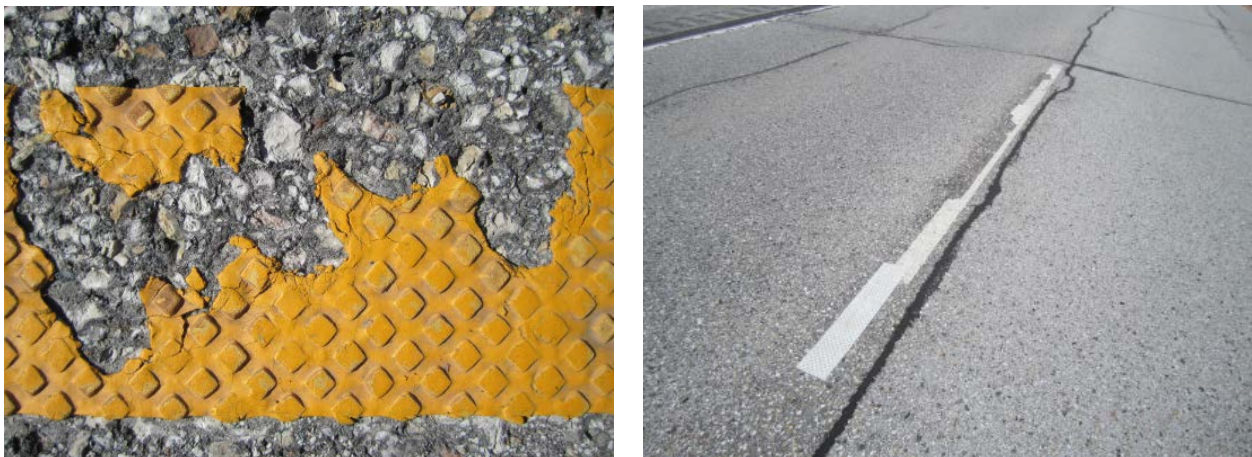
Figure 14. 3M section 11 material loss
