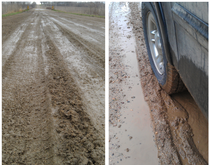
Figure 1. Examples of spring thaw conditions on unpaved roads in Iowa (pictures from Boone County on March 20, 2013)
