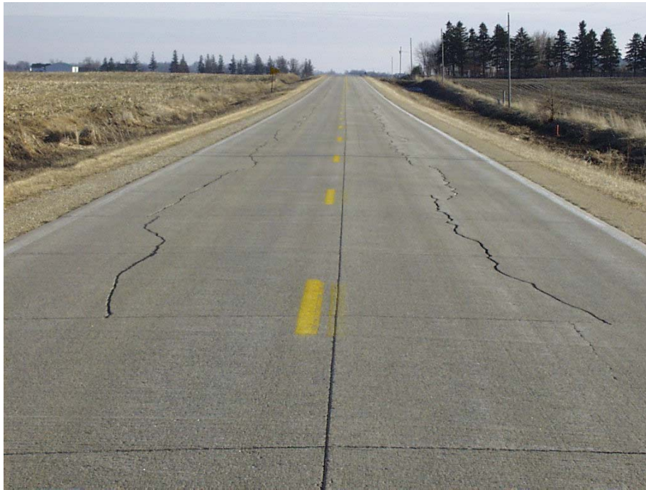
Figure 4. Picture showing a PCC pavement section in Pocahontas County, Iowa, depicting the commonly observed longitudinal cracking in relatively low-volume Iowa roads.
