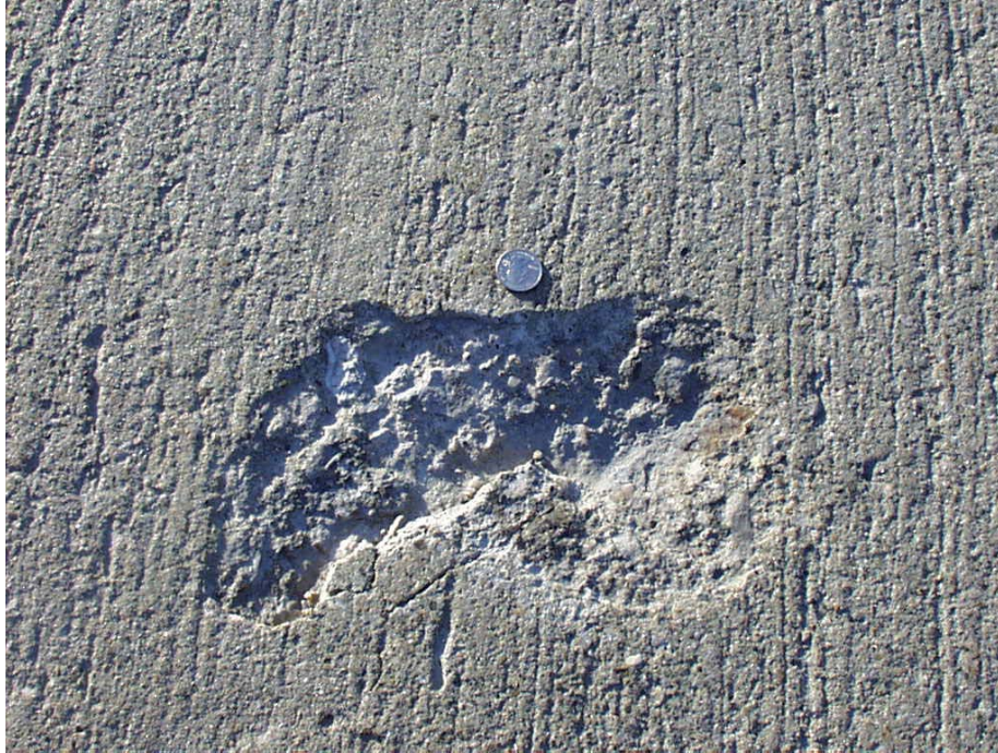
Figure 3. A view of a PCC pavement section from Marion County, Iowa, depicting the surface deterioration.
