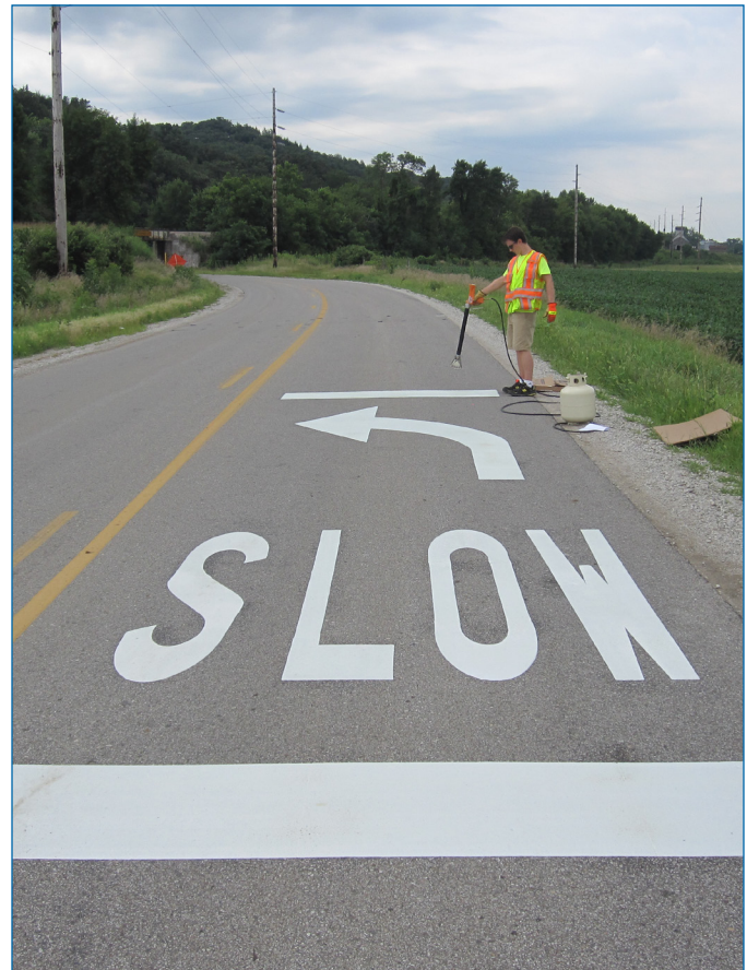
Use of a blow torch to attach thermoplastic pavement markings on CR L20
