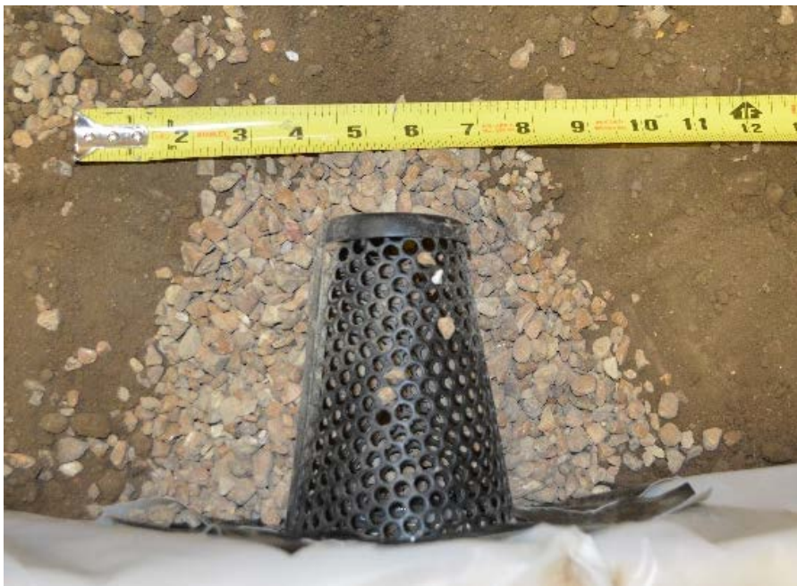
Figure 10. Back side of maintainable drain installed through center of retaining wall face during construction, with gravel placed around drain cone
