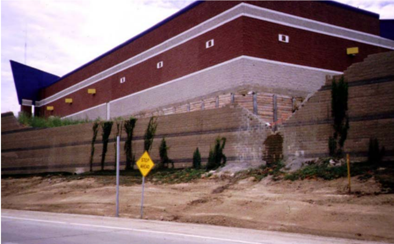
Figure 1. Failed earth retaining wall along I-70 in St. Charles, Missouri
