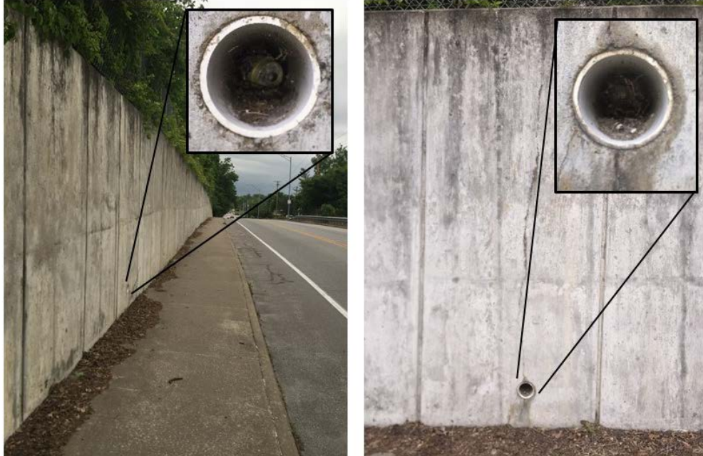
Figure 2. Questionable weep holes in cantilever wall along Old Highway 63 in Columbia, Missouri
