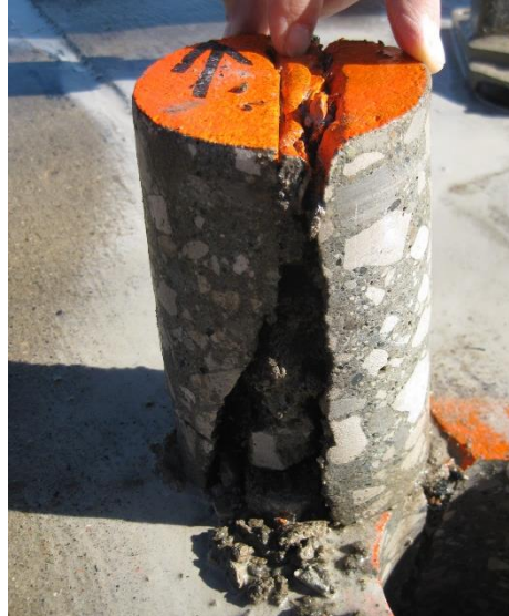
Figure 22. Core 4 taken from the distressed joint
