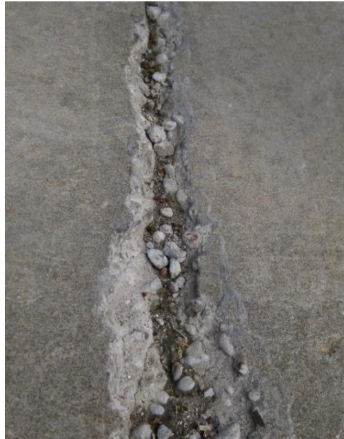
Figure 9. Field observation of joint deterioration, including exposed aggregates left behind
