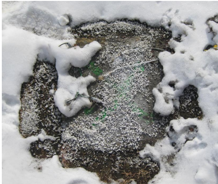
Figure 4. Sodium chloride applied on the top of the slab during a snow event
