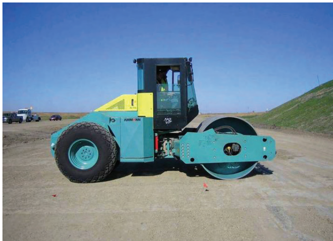
Ammann vibratory smooth drum roller with ACE system to output kB stiffness values: Field Study 2
