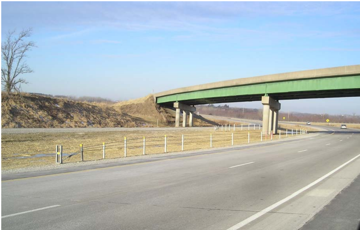
Figure I.4. High-tension cable rail in median
