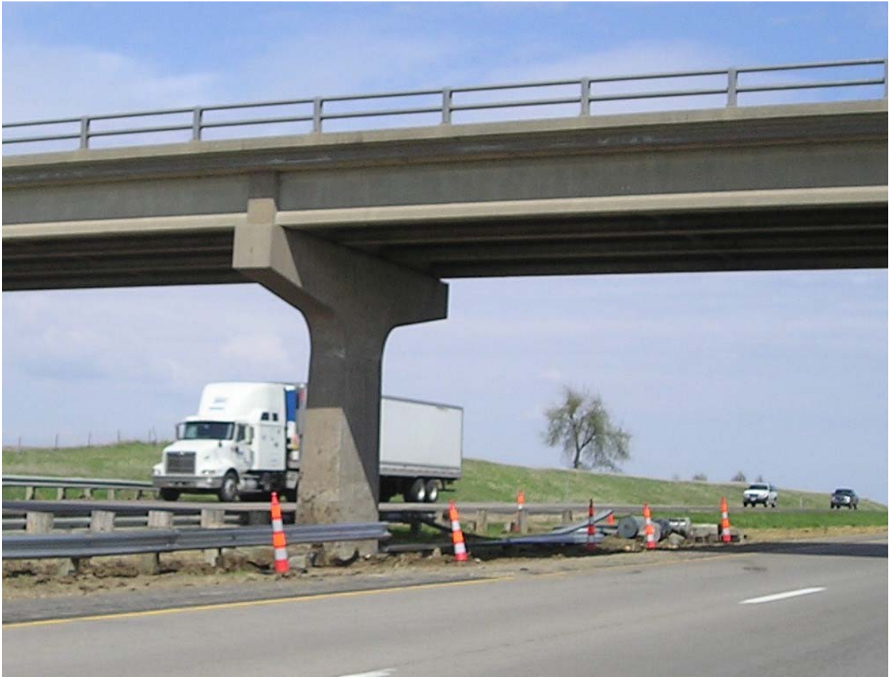
Figure I.7. Crash damage to a W-beam guardrail on I-80, May 2009
