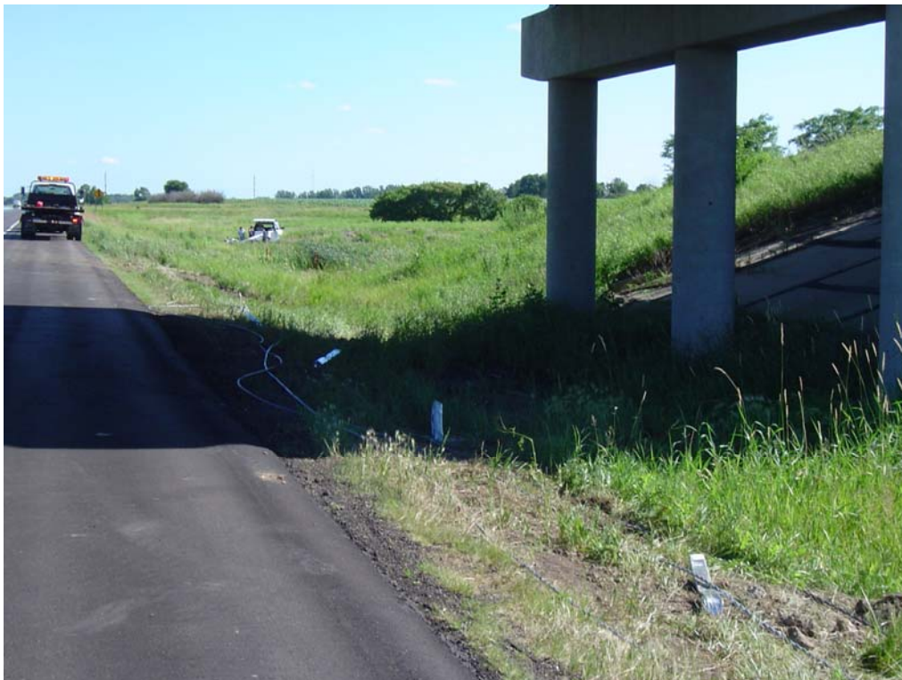
Figure I.6. Crash damage to high-tension cable rail on I-35, July 2008
