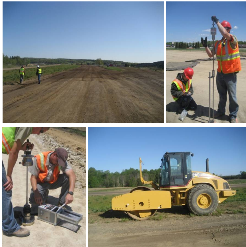
Figure 9. TB1 embankment material area and pictures of in-situ testing and roller used for mapping the area
