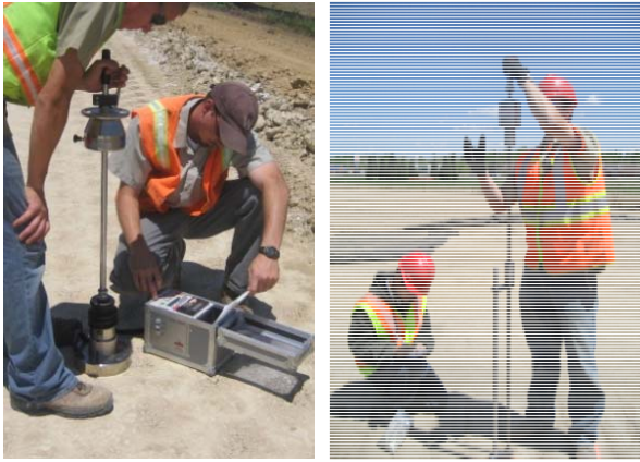
In-situ testing methods used on the test bed: LWD (left) and DCP (right)
