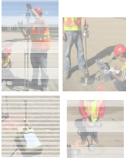
In-situ testing methods: DCP (top left), LWD (top right), Humboldt NG (bottom left), and BCD (bottom right)
