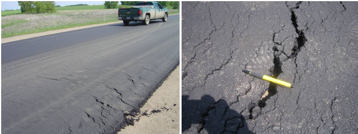
Figure 16. Premature failure observed in the HMA non-wearing course layer between Sta. 140+12 and Sta. 142+61
