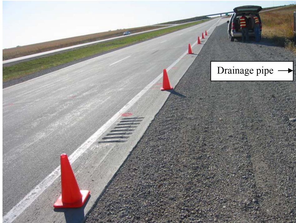
Figure 42. Pavement surface distortion, Highway 18 east (mile post 195), Iowa
