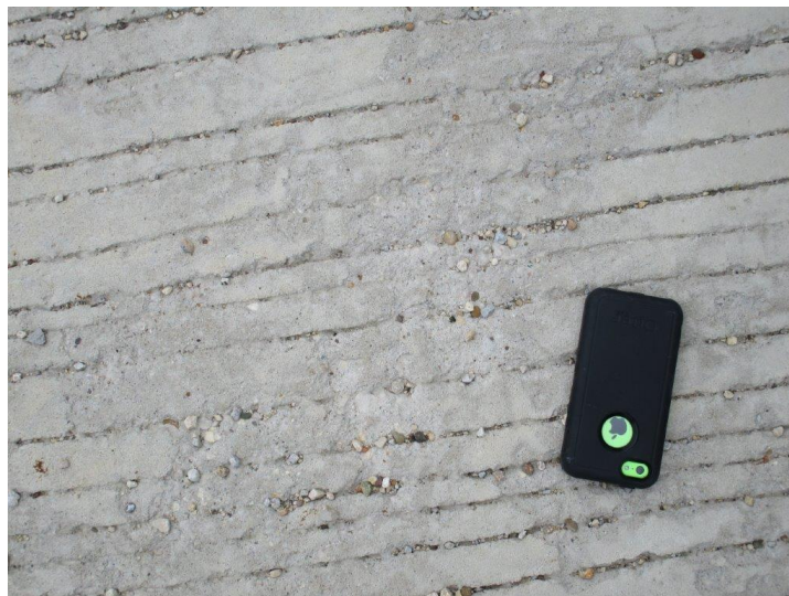
Figure 21. Limited scaling observed on the surface near drains
