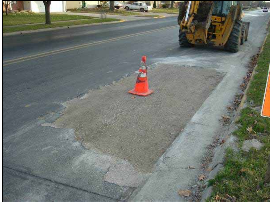
Figure 30. Utility cut left open for two weeks
