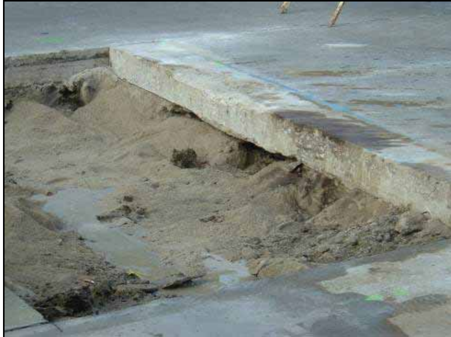
Figure 45. Backfill material caving in on trench edges
