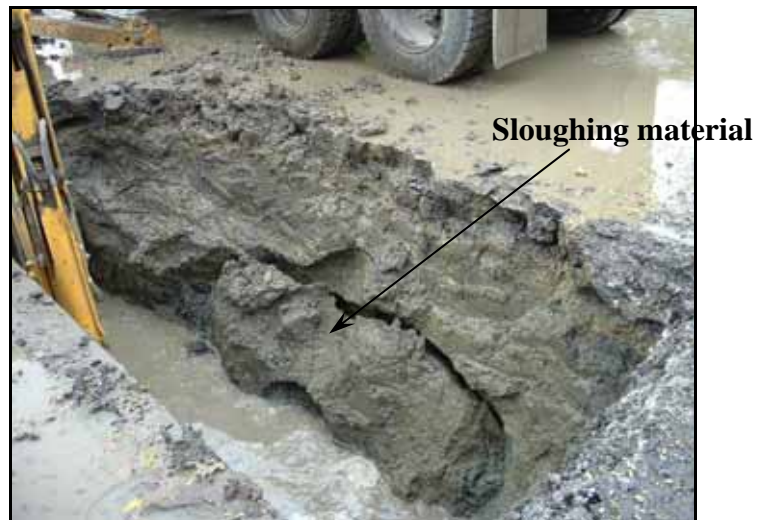
Figure 24. Material sloughing off in Ames site
