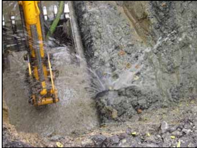
Figure 25. Ames water main break
