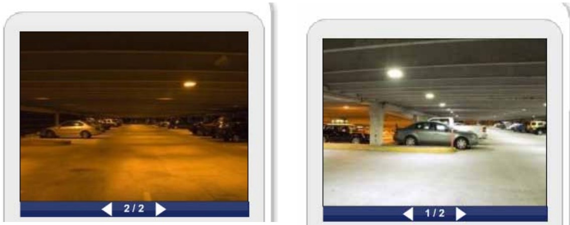
Figure 5-8: Application of LED Lighting in Parking Deck (before LED—left, After LED lighting was installed—right (Image source: WRAL, 2007)
