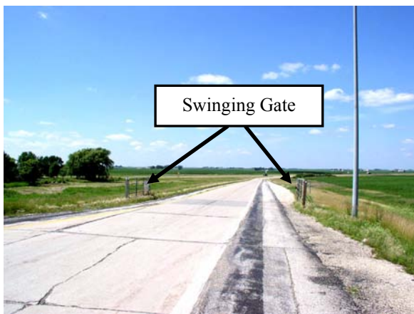
Figure 1.1. Iowa entrance ramp gates
